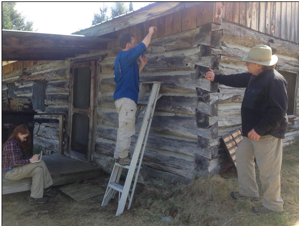
Figure 4. Sampling of the east wall at the northeast corner of the cabin. Note the newer-appearing wood above the upper tier of logs and the interlocking of logs in the corner of the cabin walls.
